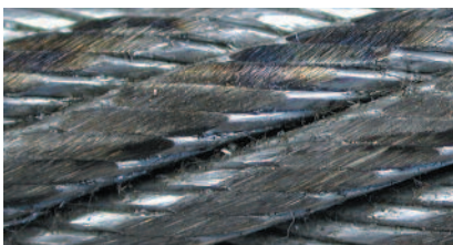
Abrasion caused by dragging the rope over a sharp object (steel corner, sharp plate, abrasive surface etc.)
